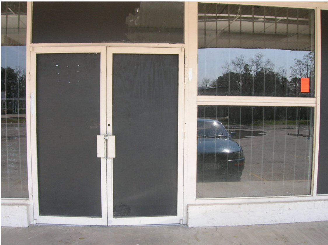
Close-up photo of 1504 Bingle showing chained doors
